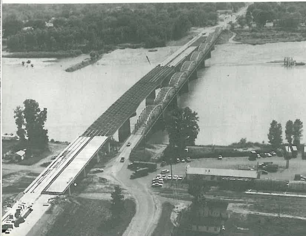
The new bridge, 4-laned and higher, dwarfs the old bridge, during construction.
